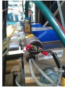
Figure 34 - The air pressure switch
