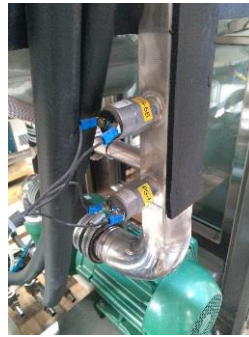
Figure 36 - The air pressure switch
