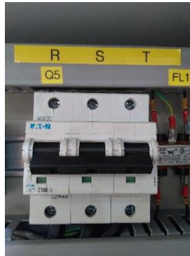
Figure 31 - General circuit breaker
